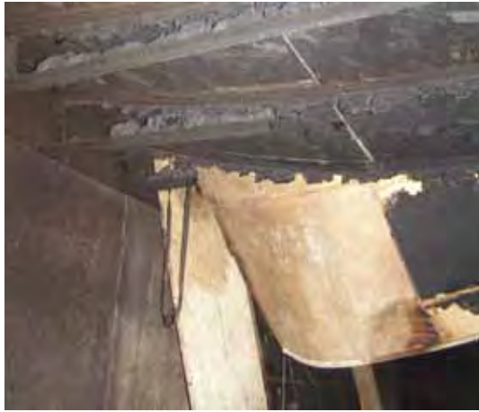
Floor assembly where Fire Engineer Arnie Wolf was killed
